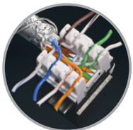
Wires held in place
